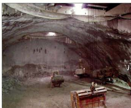
Excavation of the roof of the vast cavern to house the ATLAS experiment for CERN's LHC collider. An video on the mighty ATLAS project has just won a major award.
